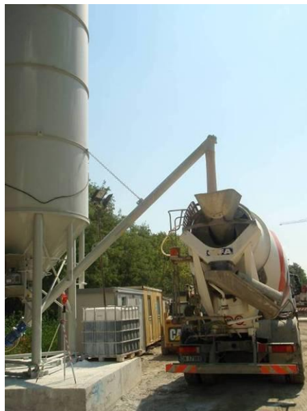
Figure 6 Supply of the expansive agent at the jobsite with an automatic silo
