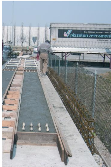
Figure 4 Field tests on restrained drying shrinkage of concrete slabs (8 m long, 400 mm wide and 60 mm thick)
